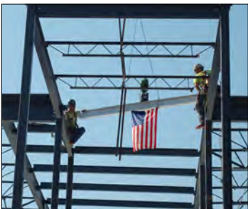
Laying the final beam atop the building after the Topping Off ceremony
